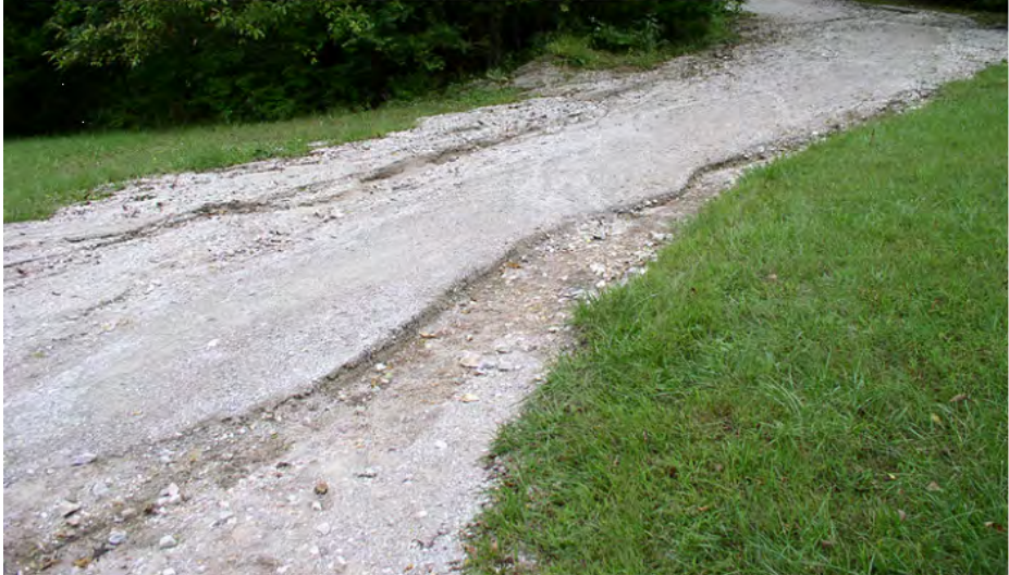
Bear Creek Trail washout after storm
