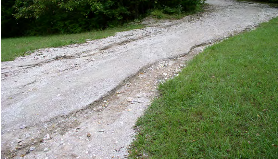
Bear Creek Trail washout after storm
