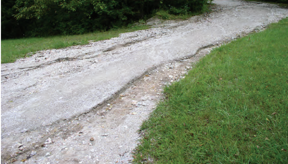
Bear Creek Trail washout after storm
